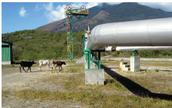
Fig. 8.4.1 Typical pipeline at Miravalles geothermal power plant, Costa Rica (photo by R. DiPippo)
